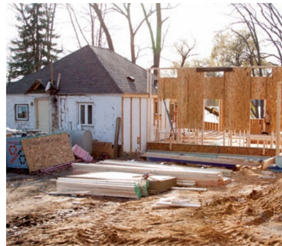
Framing work begins on an addition to the original small, concrete block cottage on Paw Paw Lake.
